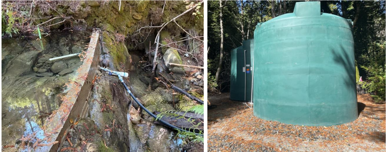
Figure 11: New intake and tanks for Waterman Gap water system
